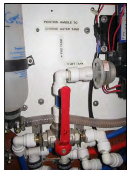
Fresh water distribution system.
