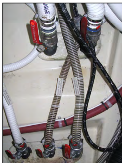
Plumbing and seacocks clearly labeled
